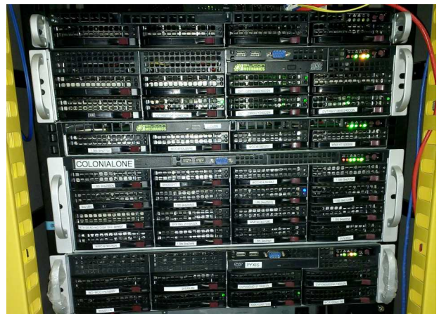
Some of the FSF's server infrastructure
