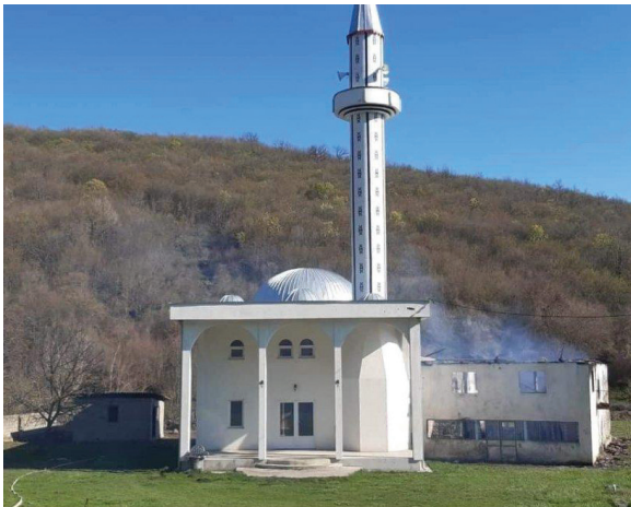
Figure 1: The burnt mosque in the village of Vërboc in Drenas Municipality. The roof and interior were seriously damaged. 12
