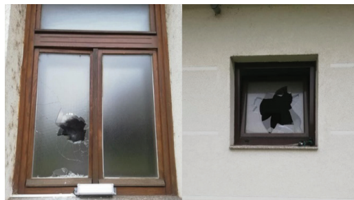
Figure 6: Shattered windows at Atik Mosque. 18
