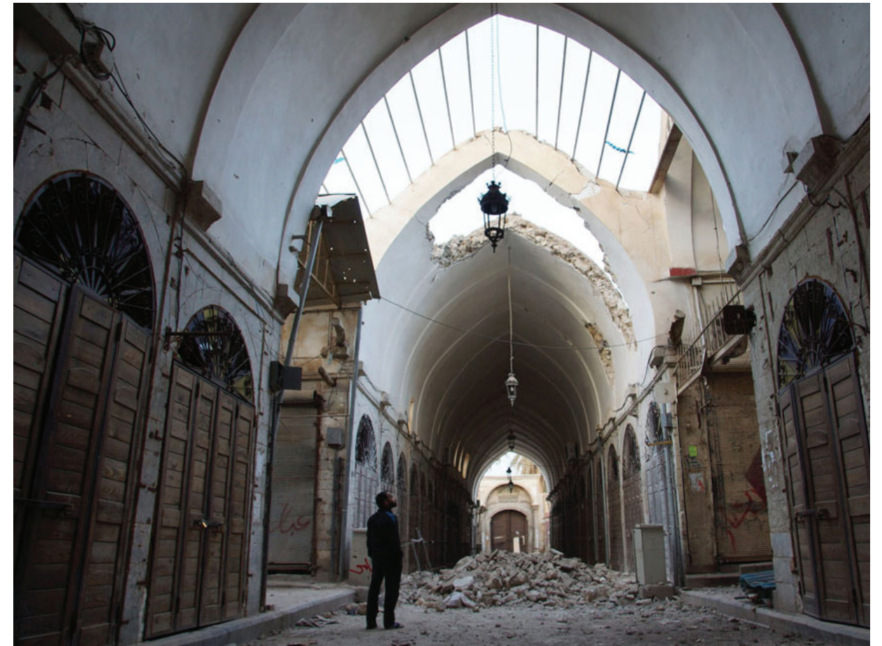
A resident inspects the damages at an ancient Souk caused, on March 9, 2013/Photo: Reuters/Khalil Ashawi.
