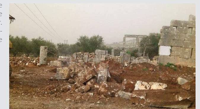
Damage to St Simeon Stylites/Photo: Directorate General of Antiquities and Museums DGAM, 2014.
