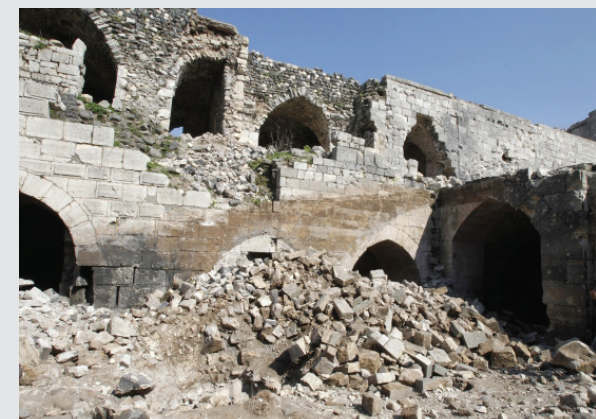
Debris inside fortification wall from collapsed stairs, 21 March 2014 / Photo: REUTERS/Khaled al-Hariri
