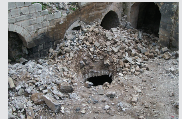
Image of the inner courtyard where the stairs have completely collapsed/Photo: DGAM, 03 July 2014
